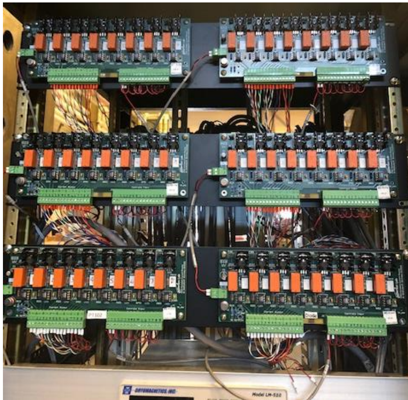
Constant current source boards #s 1-6 installed in Rack A
